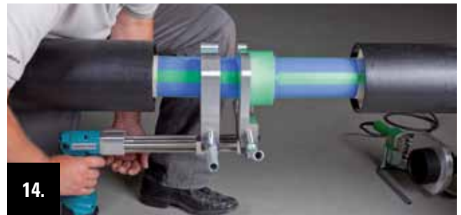
14. Drive the welding jig apart to release the fixing screw of the fitting clamping jaw.
