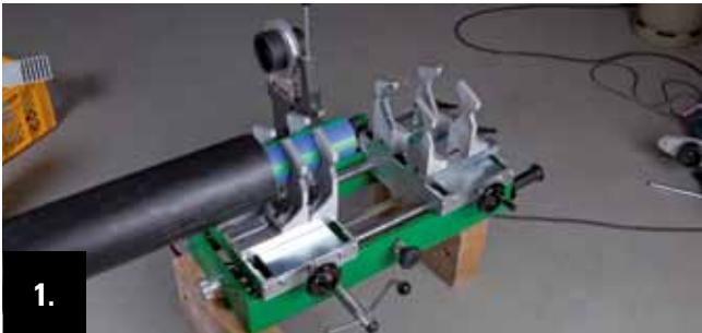
1. Position and align the welding machine. Regard the required place! (Consider that the machine must be removed below the pipeline after finishing the welding works.)
