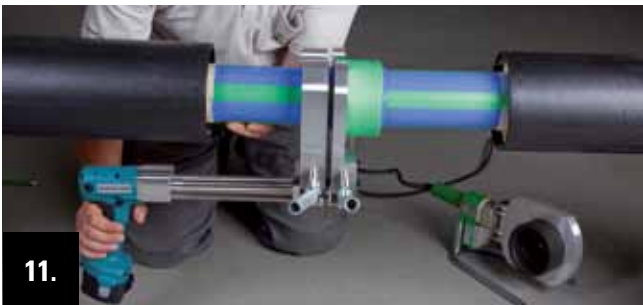
11. Press the pipe end, within the processing time, with the welding jig up to the end of the welding depth in the welding socket.
