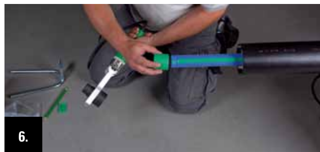
Directly after the removal of the welding device push the socket on the pipe end.
