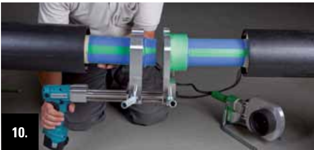
10. Immediate after removal of the welding device the welding jig is driven together slowly and evenly.
