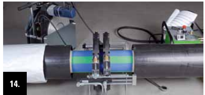
14. By using the hydraulic system the pipe ends are joined slowly until the required welding pressure is achieved.
