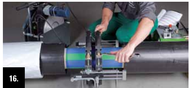
16. After the end of the cooling period the pressure is released at the hydraulic system. Then the mounting clamps are disconnected and the clamping device is removed.
